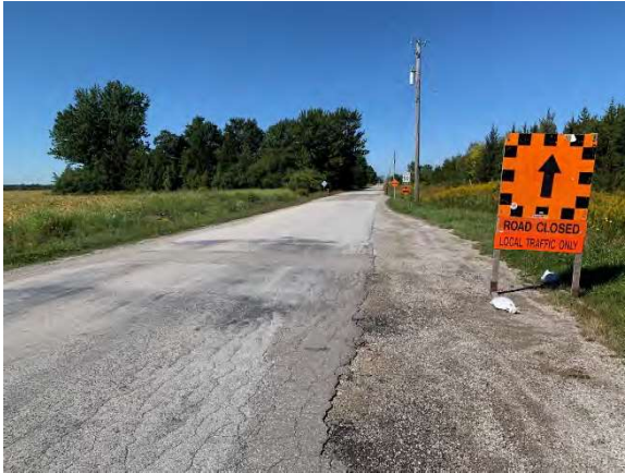
Photo 33: View of municipal road and associated disturbances, facing west
