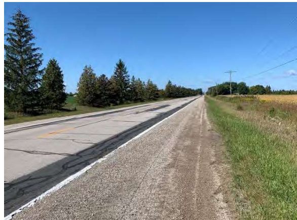
Photo 40: View of municipal road and associated disturbances, facing west
